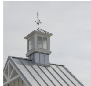
APPLICATION: Rooftop Cabinet | LOCATION: Blensburg, Maryland DESCRIPTION: 3' square, 8' tall
